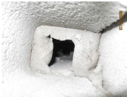
Figure 7. Photo of mortar encroaching into the grouted cell more than ½"
